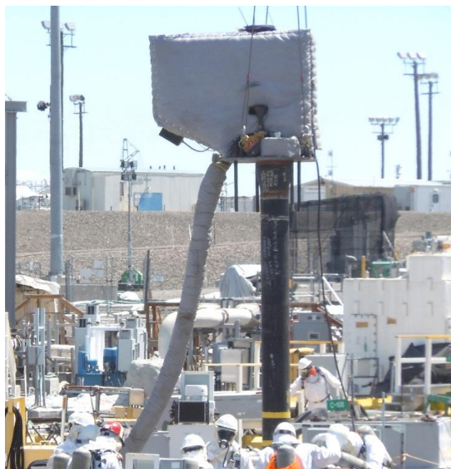
Workers install a new slurry pump in tank C-111 earlier this year to allow waste retrievals to continue. Retrieval activities were completed at the end of March. C-111 is the 15 th of 16 tanks in Hanford’s C Farm to complete retrieval activities.
