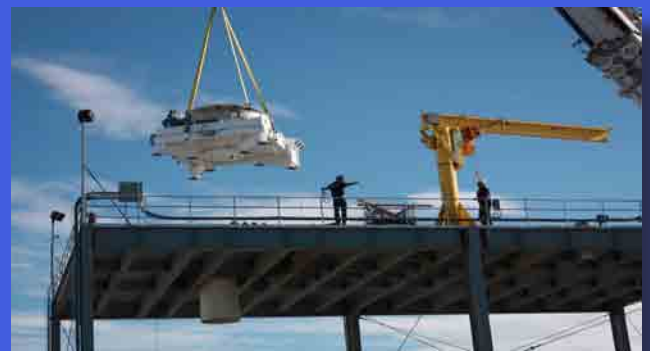
MARS turntable being installed on test stand.
