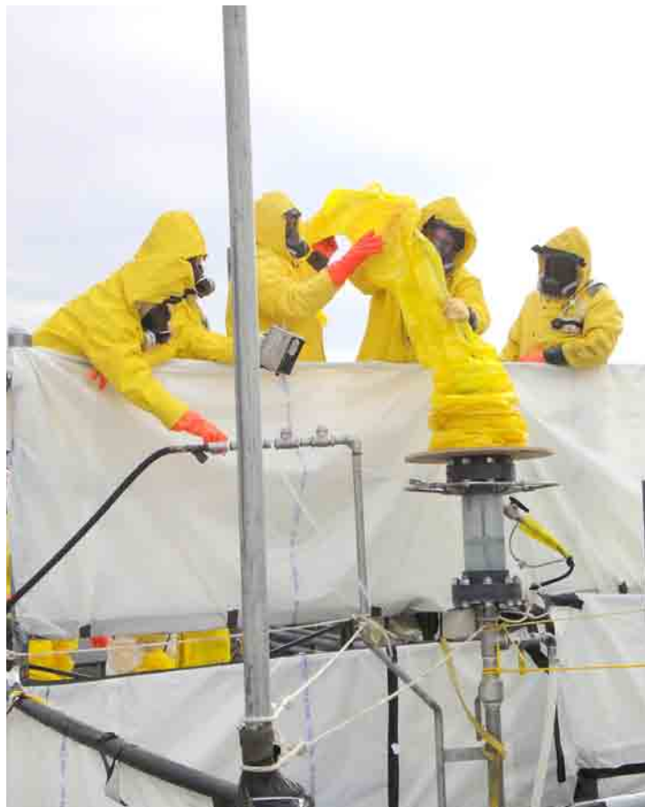
Workers contained old transfer lines in glove bags as they were cut and removed from the trenches.
