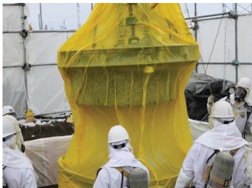
Single-shell tank C-107
