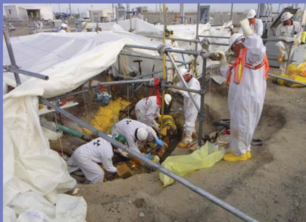
Tank waste transfer lines
