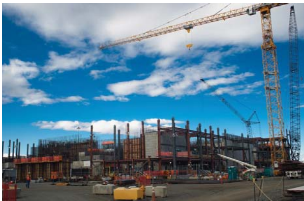
Waste Treatment Plant
