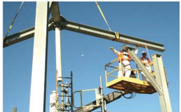
Stack extensions have been placed on two ventilation systems in Hanford's C Tank Farm to move tank waste vapors well above worker breathing space. The 23-foot extensions are expected to reduce vapor concentrations by up to 80 percent.
