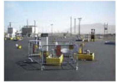
An interim barrier was installed over TY Farm. Moisture collected on the barrier is diverted to a retention basin that is filled with soil and planted with native vegetation.
