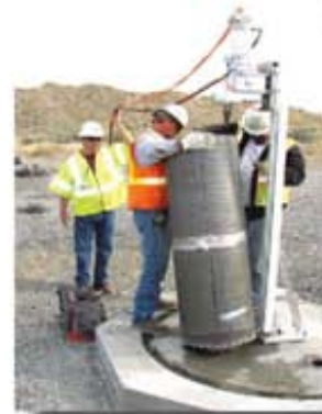
Subcontractor personnel slide a 20-inch concrete cutting bit over a riser mock-up as they rehearse for the cutting open of the dome of single-shell tank C-107 to insert the Mobile Arm Retrieval System.
