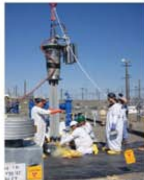
Workers successfully installed a probe into tank AW-104 to monitor tank chemistry, an important upgrade to ensure the long-term integrity of the storage tanks.
