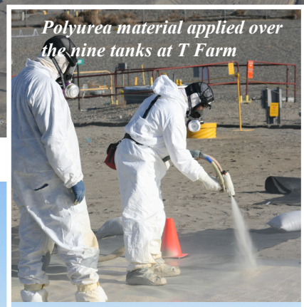
T Farm Interim Surface Barrier is made of polyurea and covers all or part of nine underground tanks.
