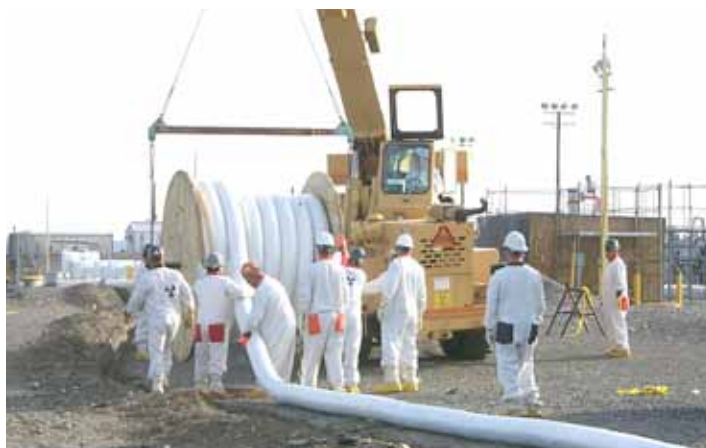
Portable hose-in-hose transfer lines are used to move radioactive waste to double-shell storage tanks.
