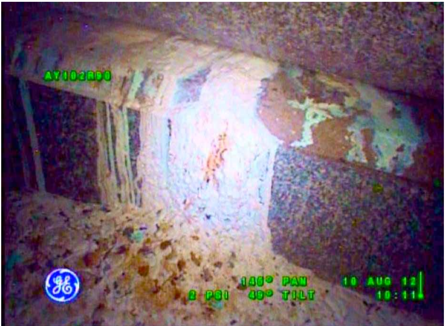
Radioactive waste is seeping from the inner shell of double-shell tank AY-102. This photo shows waste that has leaked from the primary tank into the annulus – the 30-inch wide gap between the inner and outer steel shell of the tank. There is no indication that waste has leaked outside the secondary shell of the tank.
