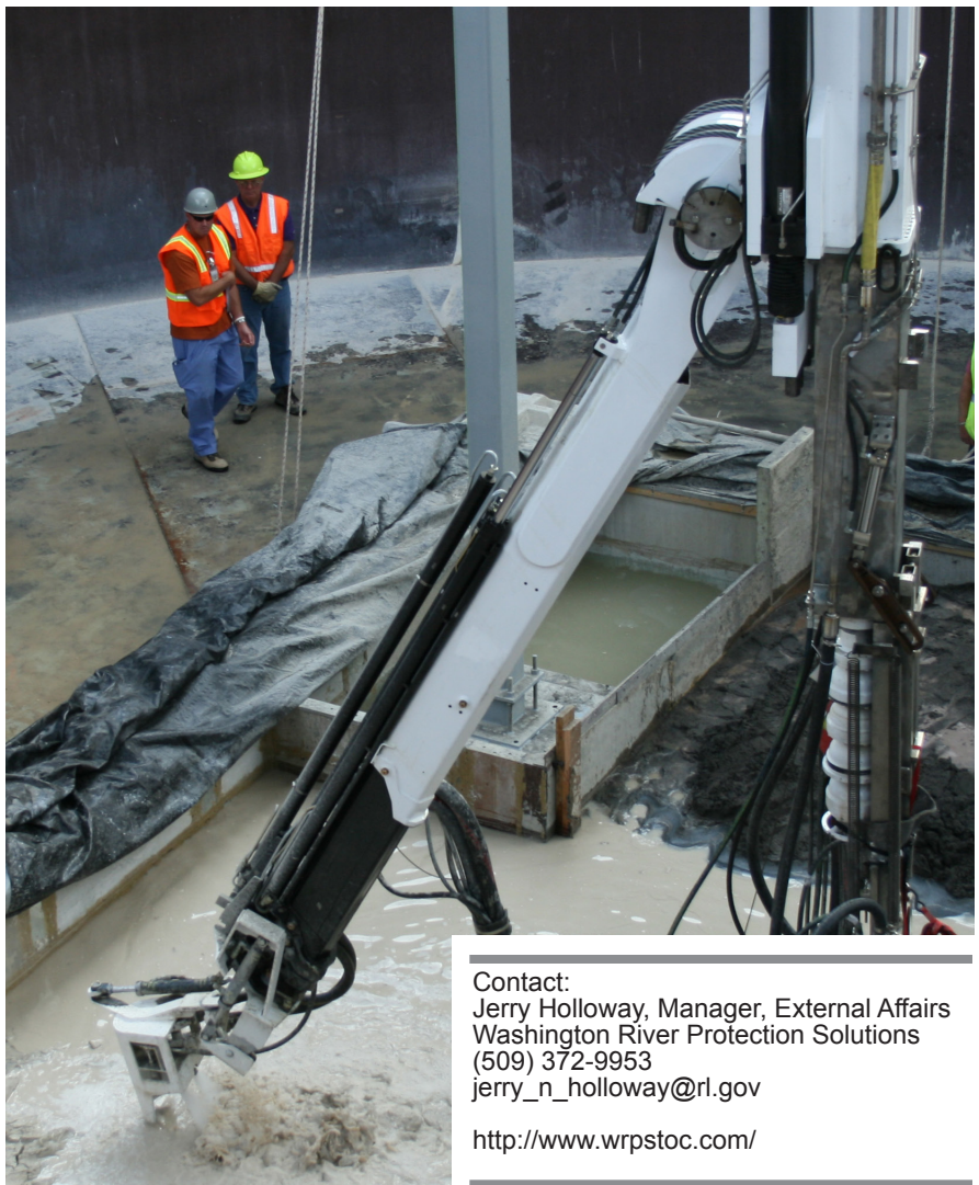
Hanford Site Cold Test Facility went into service 6/15/2002. This full-scale mockup of a single-shell tank provides a test platform for new and innovative technologies in a non-radioactive environment such as the examples pictured below.
